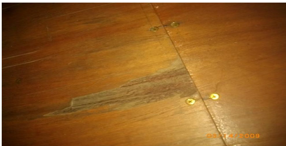
2. Small gouge on floorboard
